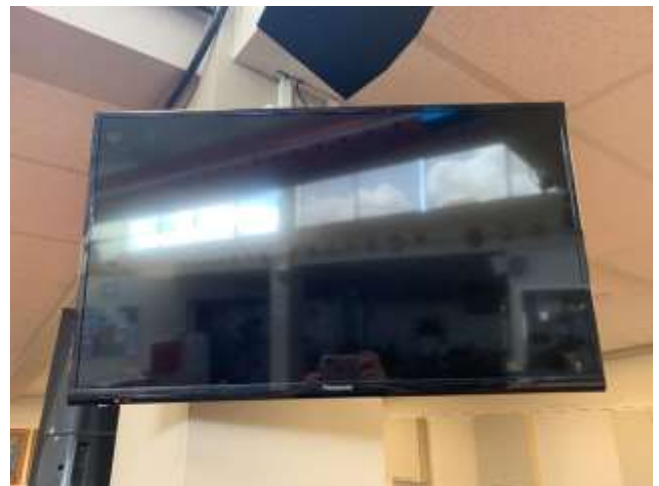
Panasonic Television 32 Inch Wall Mounted Bracket Wiring & No Remote
