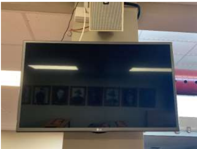
LG Television 32 Inch Wall Mounted Bracket Wiring & Remote
